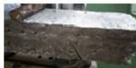
Fig 10: Crack pattern in layered beams (MC1).
