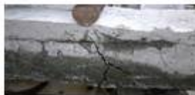
Fig 11: Crack pattern in layered beams (MC2).
