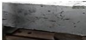
Fig 9: Crack pattern in SFRC.
