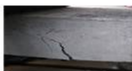
Fig 8: Crack pattern in RC.
