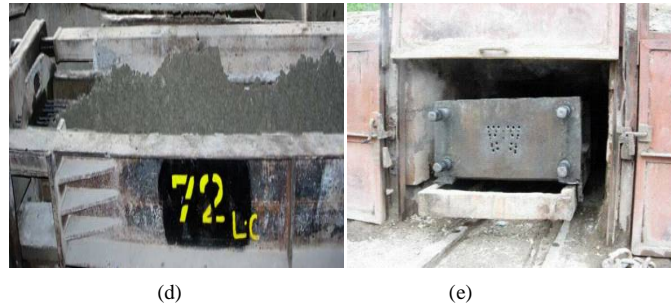
Fig. 2. Preparation of specimen (a) travelling pre-tensioning stress bench (b) a double acting hydraulic jack with a load cell (c) anchoring (d) pouring of concrete (e) steam curing chamber
