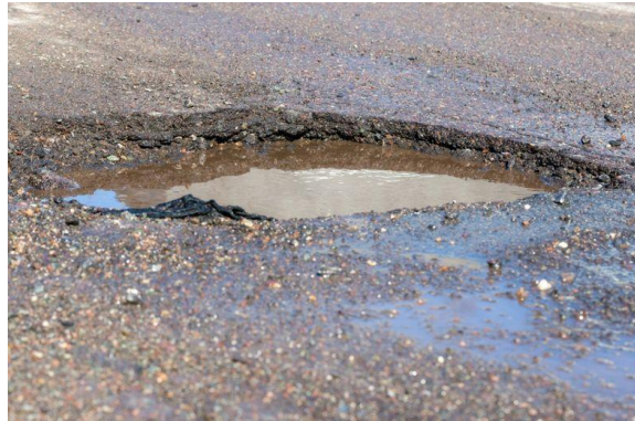
Figure 7: Pothole captured using camera
