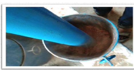
Fig 2 crushing of bricks
