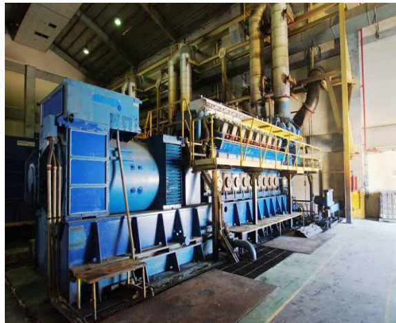
Diesel engine generator hall
