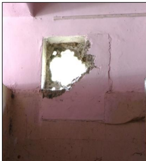
Fig.6 Broken toilet ventilator
