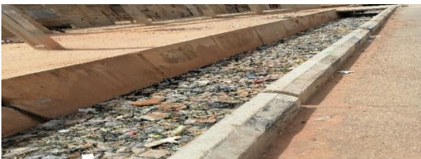
Fig 5 Drainage facility in Adamu Aleru Estate
