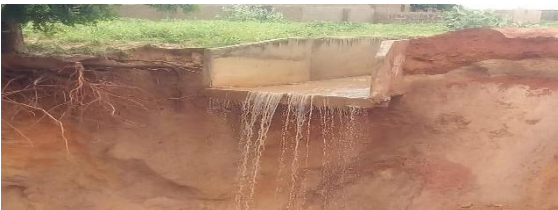
Fig 7 Drainage facility in Tudunwada area
