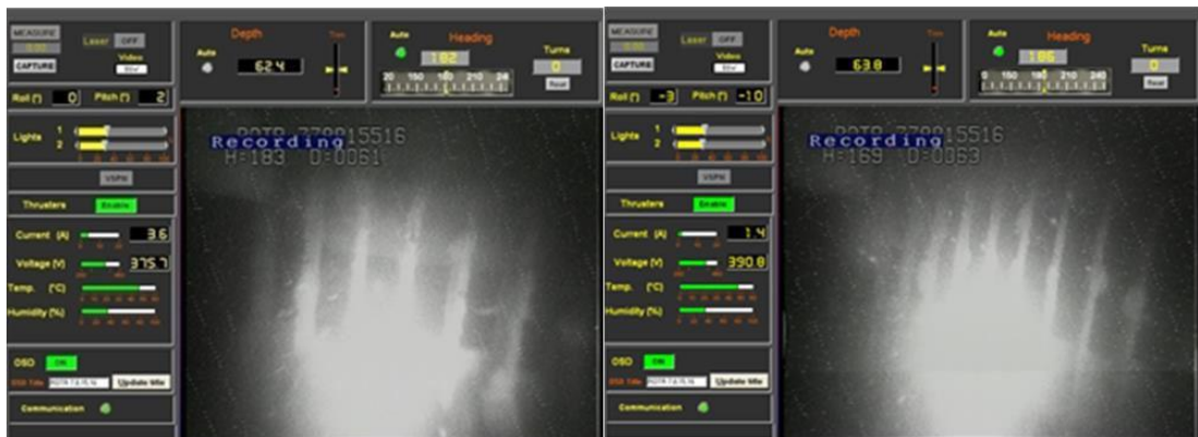
Fig. 7. Steel bars of river outlet trash racks after partial removal of silt.
