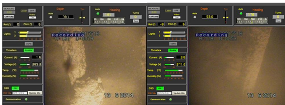
Trash rack of river outlet at 79 m depth Trash rack of river outlets at 53 m depth
