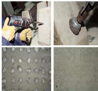
Figure 1 A) Substrate surface partially chipped, B) Substrate surface prepared with steel brush
