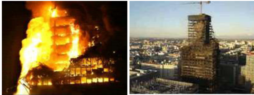
Fig.1. – The Windsor Tower’s fire, Madrid (2005): a) full developed fire, b) post-fire damaged structure .
