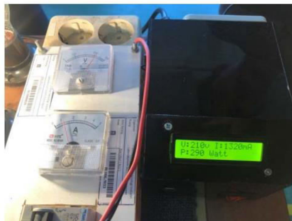
Figure 4. Current sensor testing
