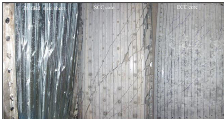
Figure 6: Failure mode of steel sheet and concrete core under monotonic loading.
