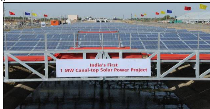
Fig 4. Solar panels above the Narmanda irrigation canal
