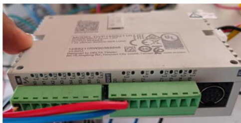
Fg No.2.4. 1.DELTA-PLC (Programmable Logic Control)
