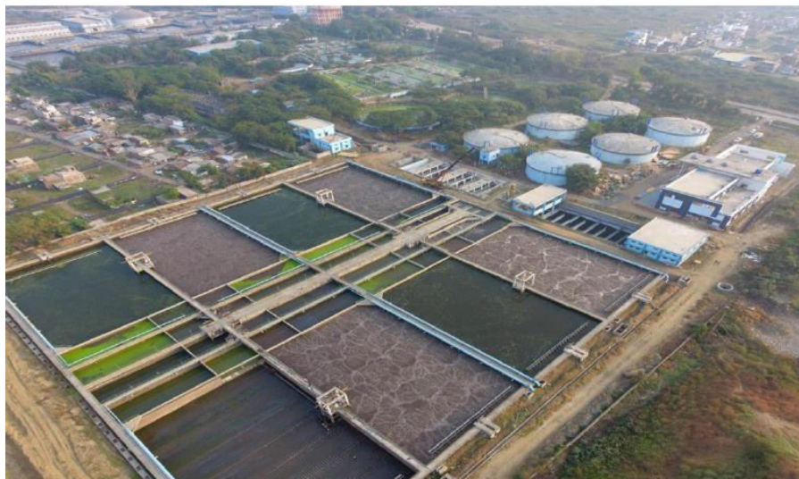
Pic 1: Water Treatment Plant
